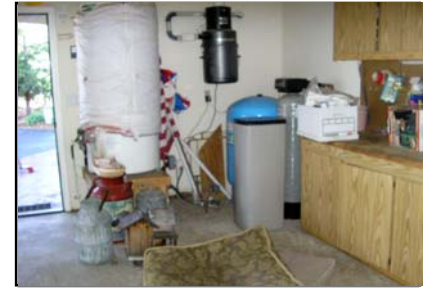
Water equipment located in garage.
