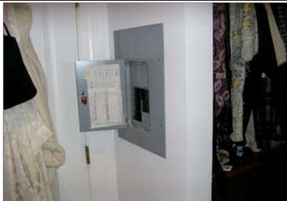
Sub panel located in master closet.
