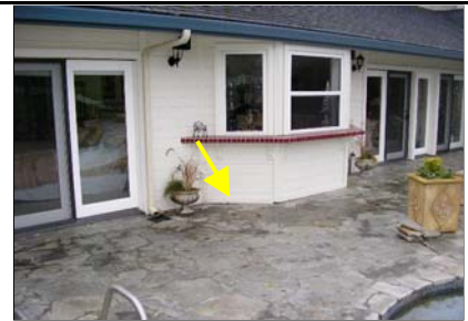
No clearances noted along rear siding material.
