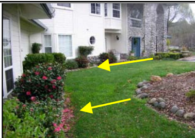
Negative grade noted towards front of house.
