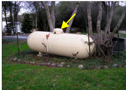
Main gas shut-off at tank.
