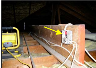
Exposed wiring noted in garage attic.
