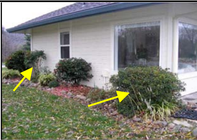
Recommend trimming vegetation away from siding.
