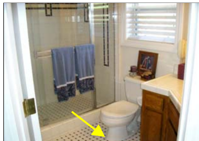
Bathroom # 2 - toilet not secured to floor.
