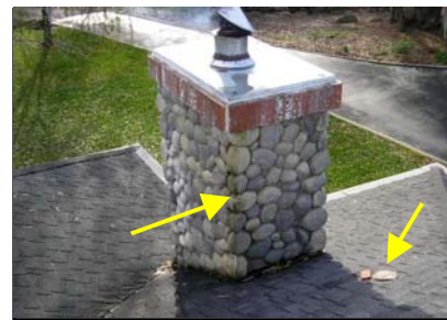
Right chimney - cracked veneer noted, missing brick noted. Ponding water noted on cap.
