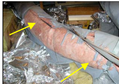
Deterioration noted to duct vapor covering
