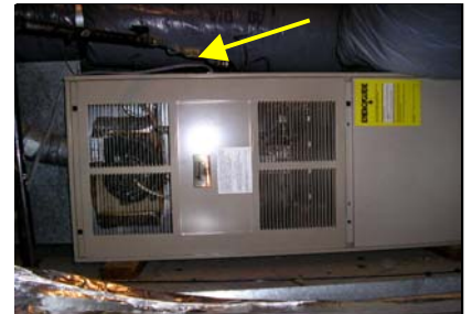
Gas shut-off valve - upper attic unit.
