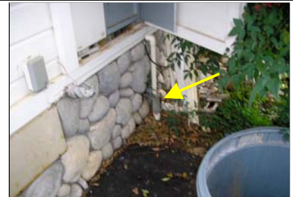
Exposed wiring in junction box below main panel.
