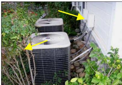
AC condensers & disconnects. Vegetation contacting units.
