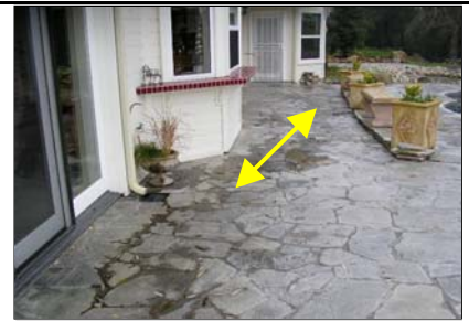
Ponding water noted on stone patio behind house.
