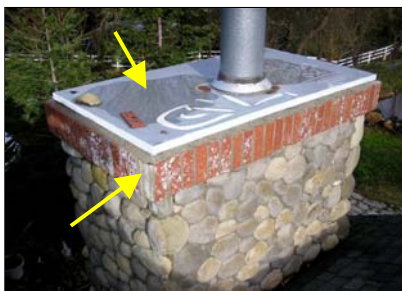
Left chimney - cracked veneer noted, missing bricks noted. Ponding water noted on cap.
