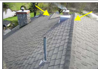
Recommend caulking exposed nail heads along ridge cap.
