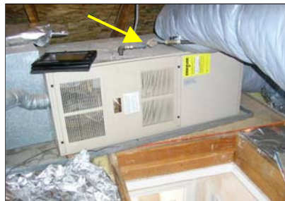
Gas shut-off valve - lower attic unit over master bathroom.
