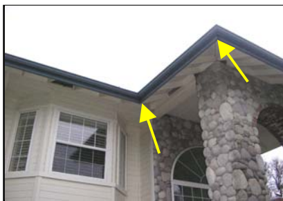
Dripping noted at front gutter corners.
