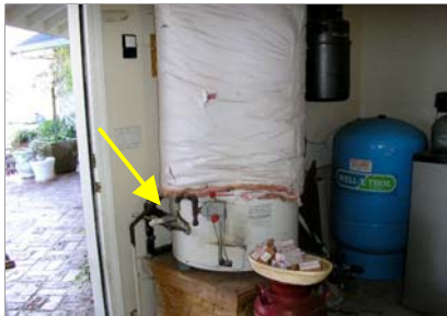
Water heater gas shut-off valve. No EQ strapping noted.
