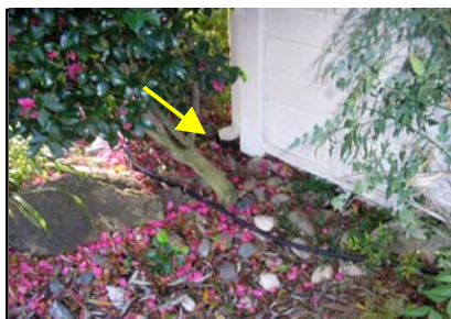
Recommend extensions on all downspouts.
