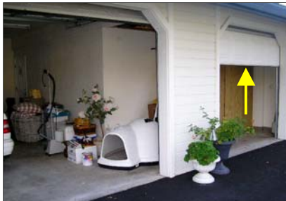
Right side garage converted. Garage door hangs up on office framing.
