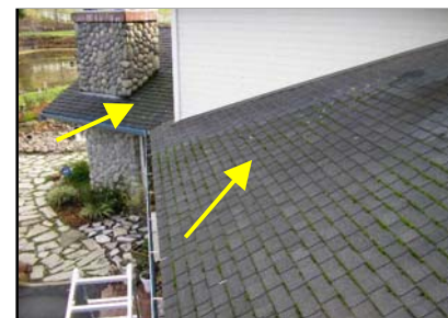
Moss build-up noted on rear/ north side roofing.
