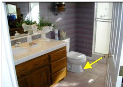
Bathroom # 3 - toilet loose.
