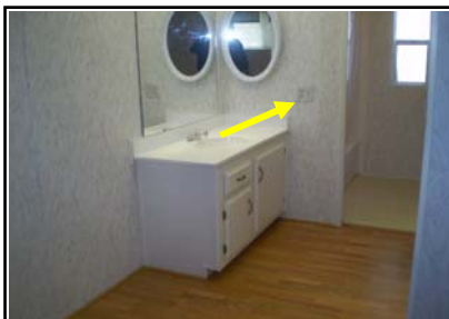
Master bathroom sink outlet is not GFCI protected.
