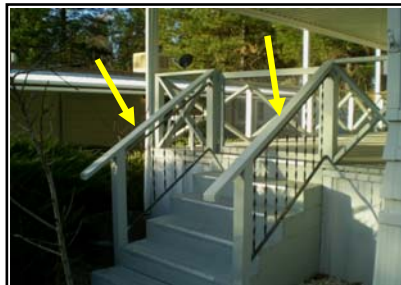
Graspable hand rails are not present at deck steps.
