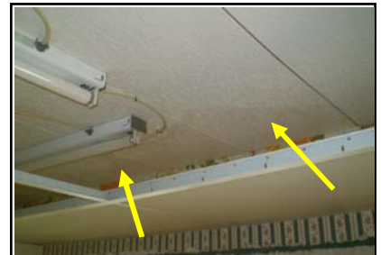
Staining noted to ceiling over sink area.
