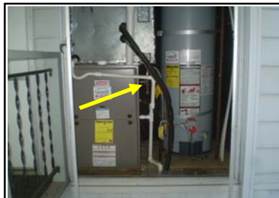
Exterior closet - furnace gas shut-off valve.
