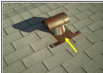
Rusting noted to vent pipe flashing.
