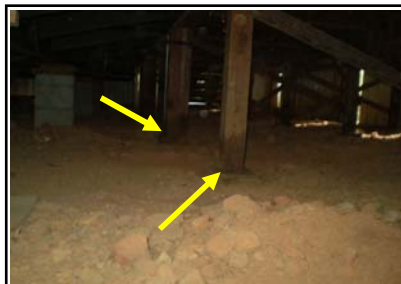
Earth to wood contact will accelerate wear to post material.
