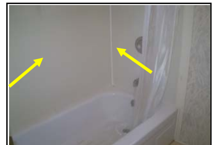
Individual single sheet panels noted in shower will leak if not maintained.
