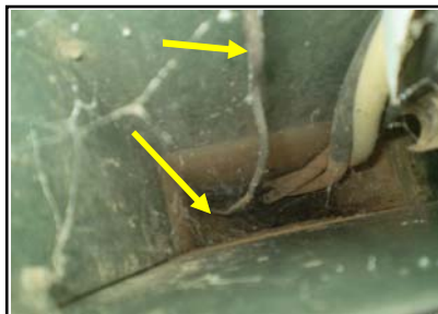
Electrical panel ground wire disappears into soil in bottom of panel.
