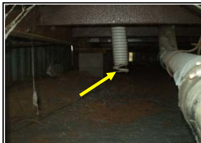
Dryer debris is discharging into crawl.
