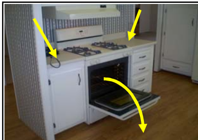
Stove anti-tip brackets are not installed. Counter tops are not secured to cabinet.
