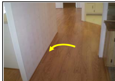
Unlevel flooring noted in center hallway.
