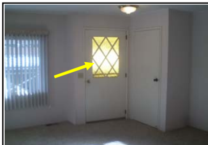
Front entry door glass is loose, rattles.
