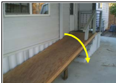
No railing & high edge noted off side of ramp.
