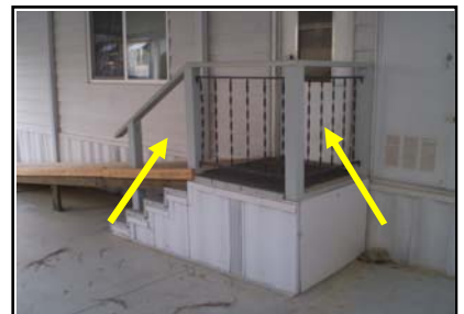
Porch railing openings are insufficient for small children.
