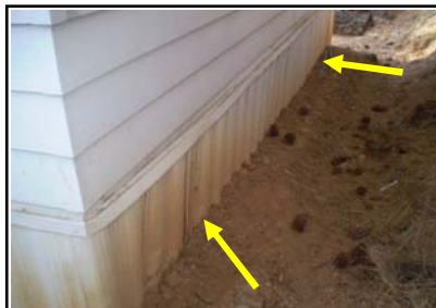
Wear noted to skirting material at soil contact.
