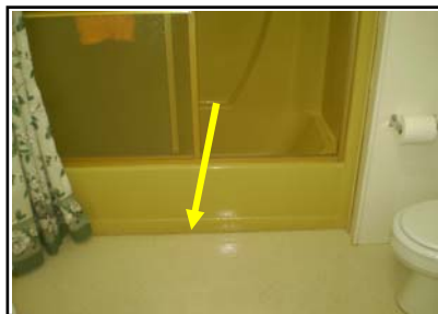
Recommend keeping tub seams/ edges caulked/ sealed.
