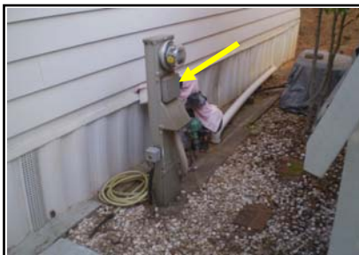
Main electrical disconnect is located at pedestal.
