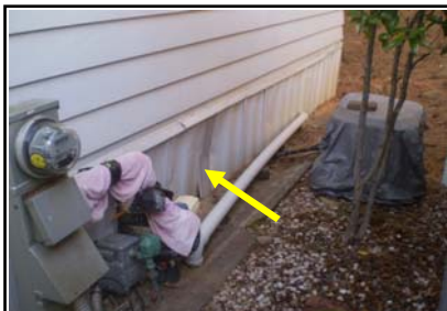
Skirting material bent, dented.
