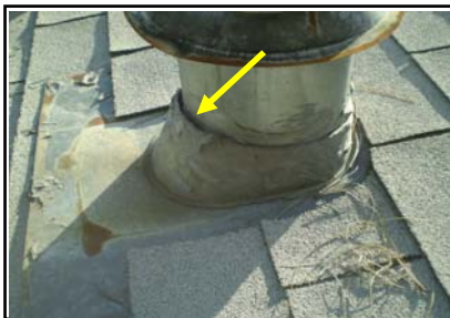
Gaps noted in vent pipe flashing sealant. Staining noted to water heater closet ceiling under flashing.
