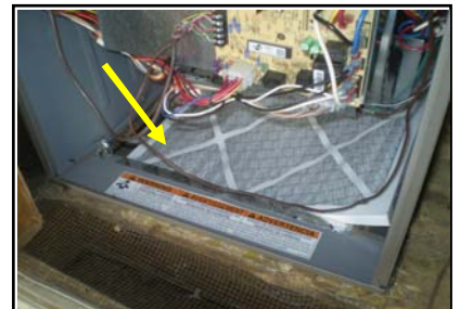
Return air filter in furnace has collapsed.
