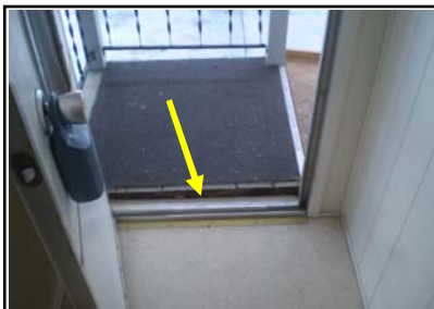
Uplifted edge noted out of right side entry door.
