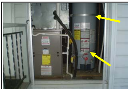
EQ strapping is not securing water heater from movement.
