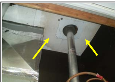
Staining noted to water heater closet ceiling.
