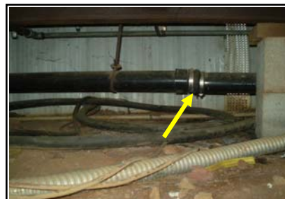
Leaking noted at drain line flex connector under house.
