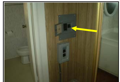
House breaker panels are not recommended to be in clothes closets.
