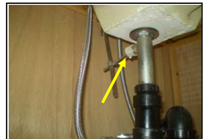
Leak noted at sink drain stopper assembly under sink.
