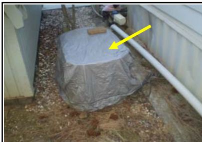
No electrical disconnect noted at AC condenser.
