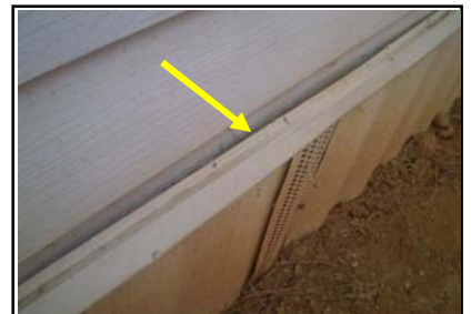
Loose skirting trim material noted.
